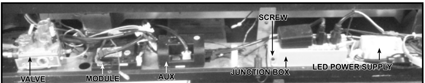
Figure 8.4. Valve Cavity (Lower Access Cover Panel Removed)
